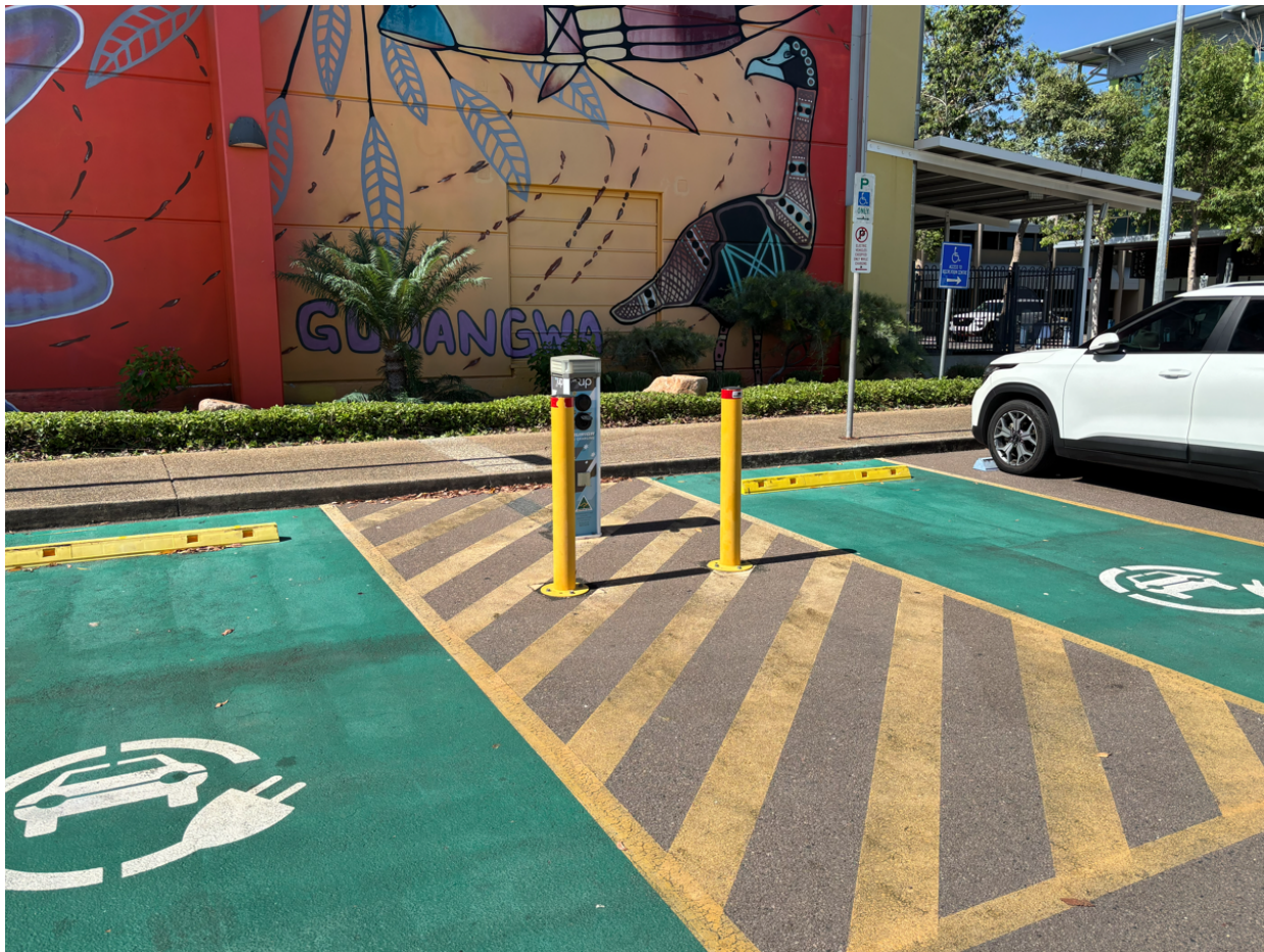
Figure 1: EV charger, Palmerston Recreation Centre car park
