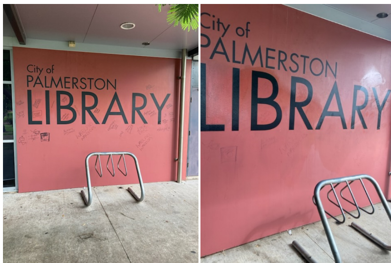
Figure 16: Graffiti removed at Palmerston Library, restoring a clean and welcoming facade for the community.
