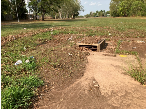
Before: Moulden Drain pit 92 and apron
