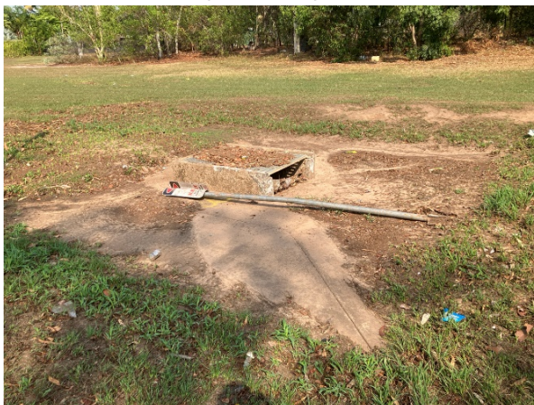
Before: Moulden Drain pit 93 and apron
