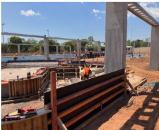
First structure complete for leisure pool and shade structure steel above columns 06/09/23
