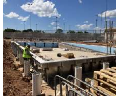
Program pool showing Myrthra gutters 06/06/23
