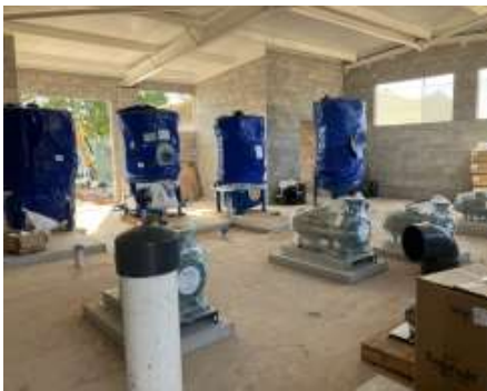
Internal plant room equipment installed 06/06/23
