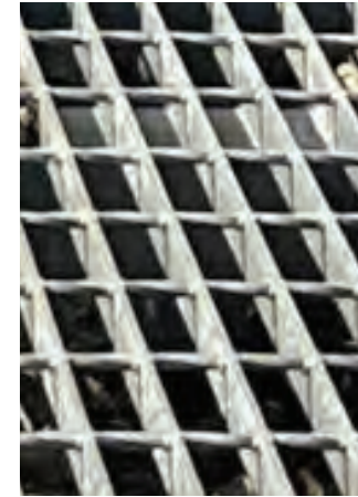
CREEK CROSSING OR AREAS OF INUNDATION - STEEL GRATE DECKING
