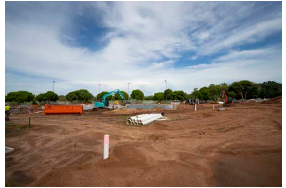
Work on Palmerston's aquatic precinct starts from the ground up with essential groundworks.
