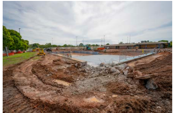
Demolition of the old pool is well underway and construction is currently on-track.
