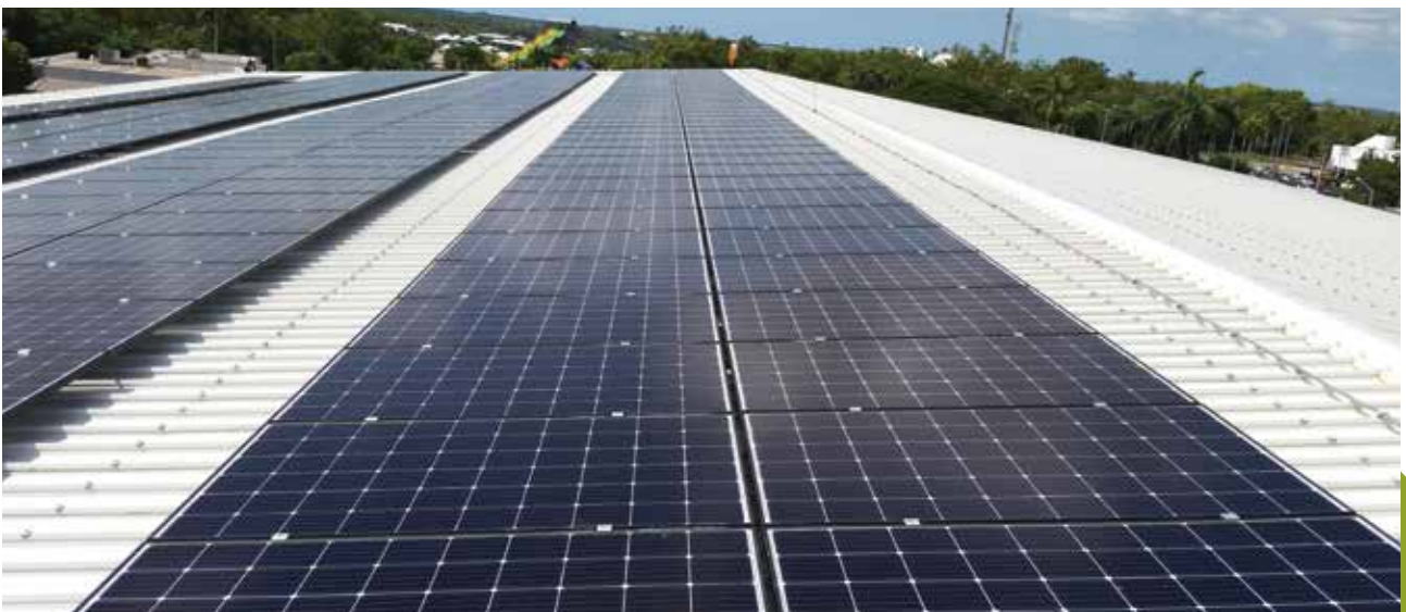
Above: Solar panels on Palmerston Recreation Centre.
